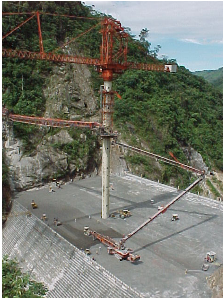
Example of all conveyor delivery system
