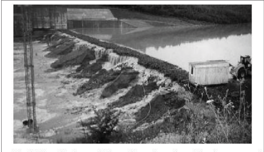
The picture shows water seeping above the top of the core.
