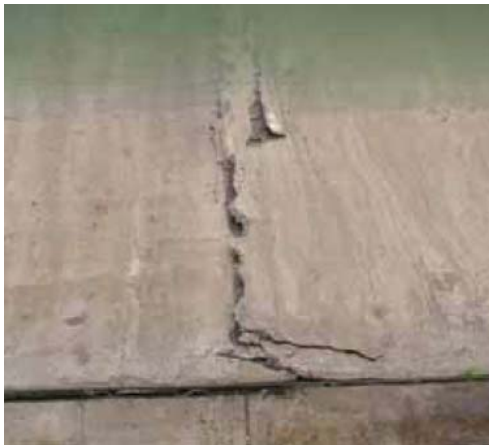
Figure 1: Crack seen from above between slabs 17 and 18
