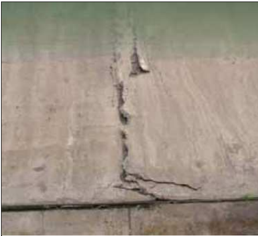
Figure 4: Crack seen from above between slabs 17 and 18 (Ref [3])
