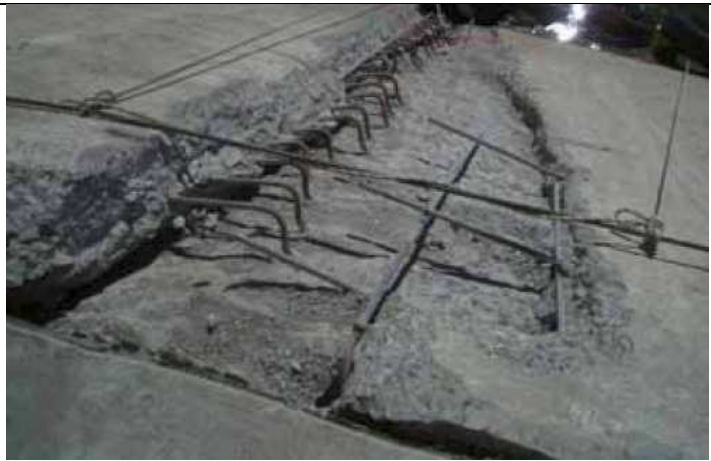
Figure 5: Slabs 17 and 18 after removing sheared concrete (Ref [3])
