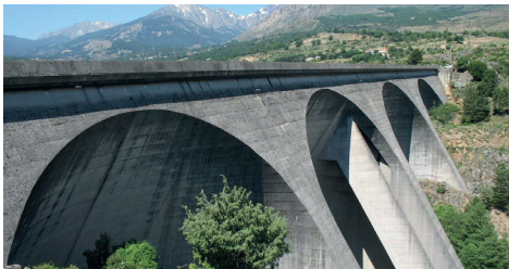
Credit photo : Calacuccia operator EDF
